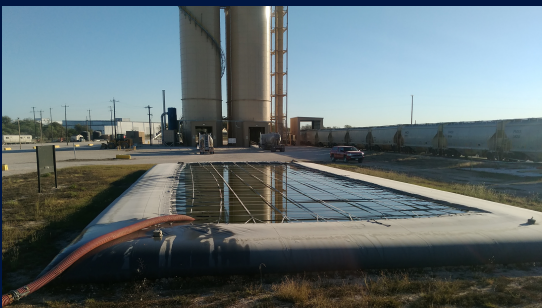
FlexSS being used to contain slop water at Southton Railyard in San Antonio, Texas
